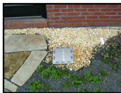
(6) Common Green Roof Drains
