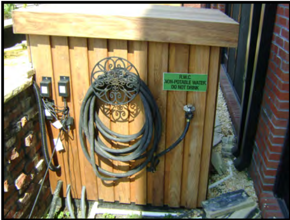
(18) Main Green Roof Hose Bib
