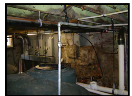
(14) Fresh Water Supply
